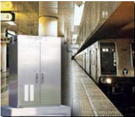
Pad mount ASAP V/CIP system node
