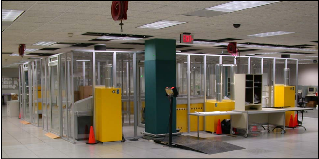
Installed Negative Pressure Mail Room (NPMR).
