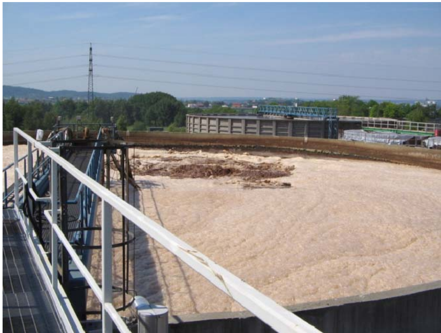
Figure 1.1. One of the aeration ponds at the biological treatment plant at Borregaard Ind. Ltd. (Photo: FFI).
